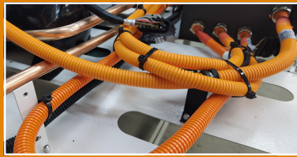
High Voltage Connection
