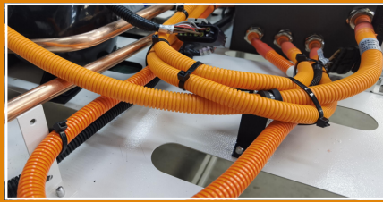
High Voltage Connection
